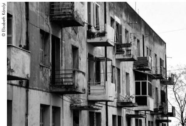
Fig. 6. Façade looking onto Alexandras Avenue: most of the inhabitants have been evicted, Spring 2004
